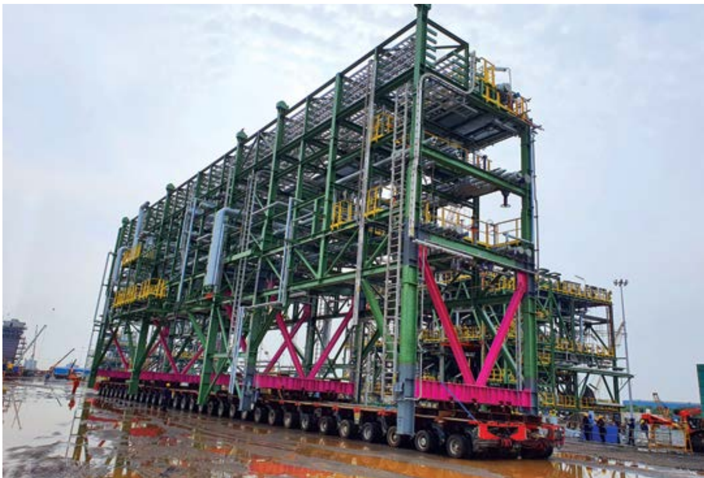
Singapore Gasification Modules - Linde
